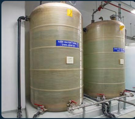
RAW WATER TANKS
